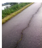
Scheurvorming asfalt Diemerpark (B)
